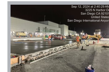
P-501 Concrete Placement using the Allen Paver with the RTP 500 Placer in San Diego Airport
