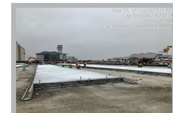
First Placement of Lean Concrete Base on Ph 4 at MSC South in LAX Airport
