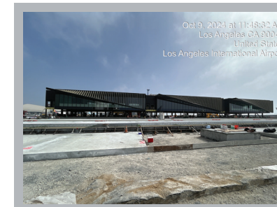
Progress photos of Lean Concrete Base and P-501 Pavement placed at the MSC South in LAX Airport
